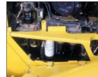
Additional main fuel filter
